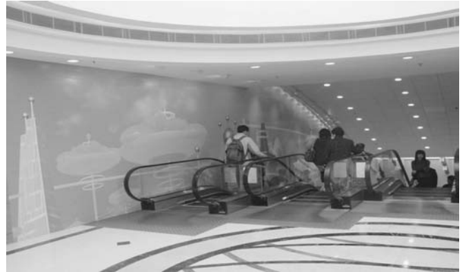
Figure 1 High Speed Escalators at MTR Station.
